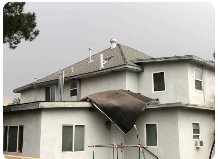
Roof damage in Highland Park
